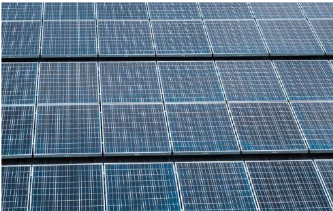
SOLAR POWER PLANT, Kangra, Himachal Pradesh
